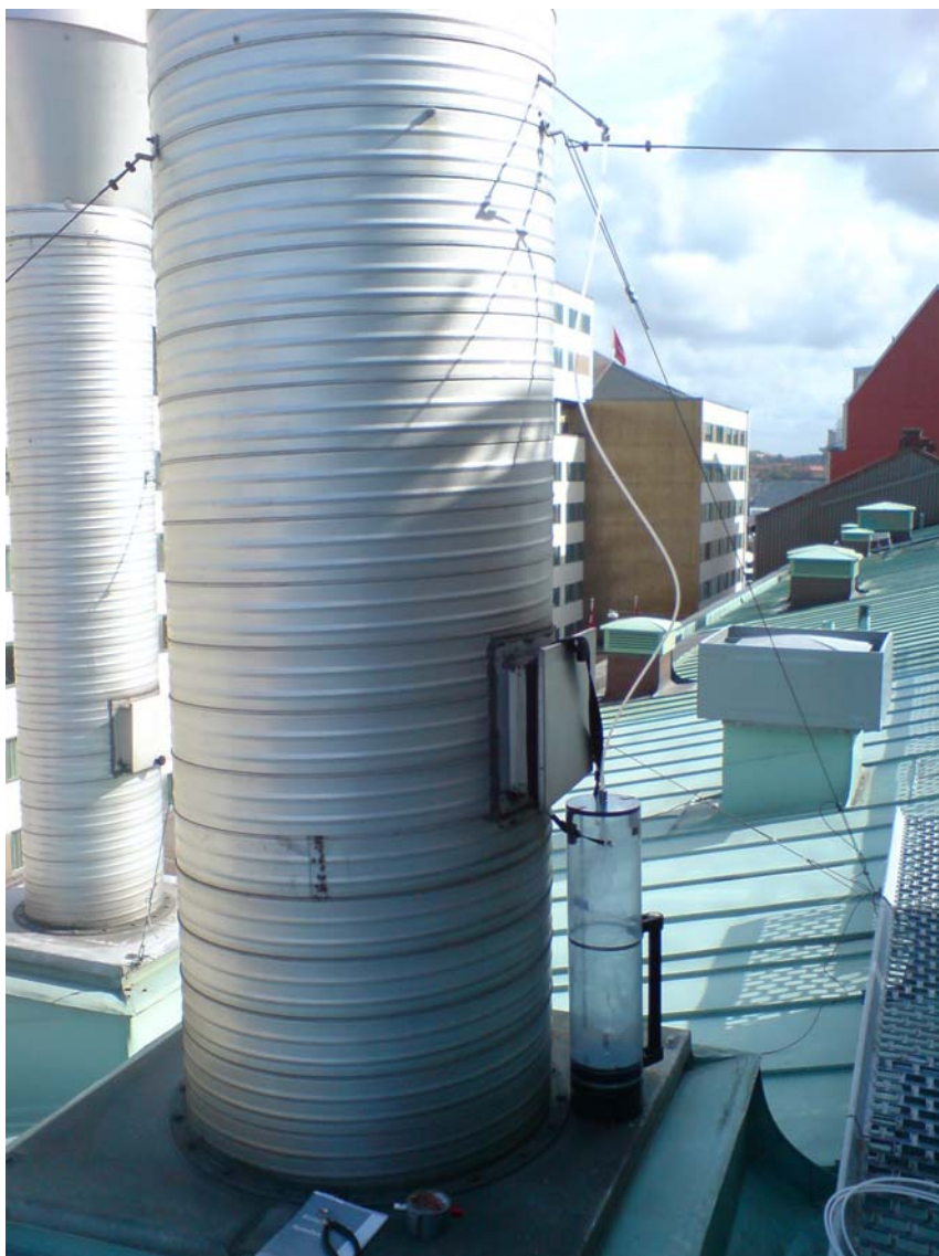
Figure 1 Odour sampling after the fan unit.
